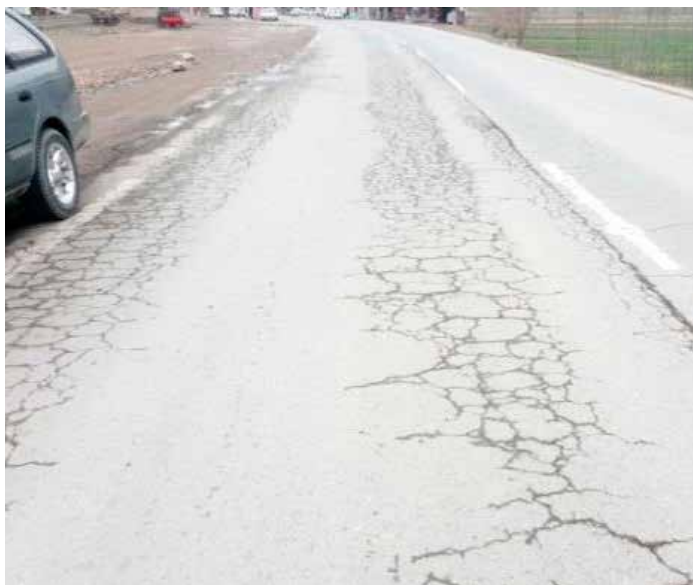
Cracks on Surface of the Road
