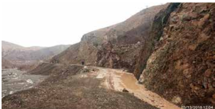
Lack of Drainage
