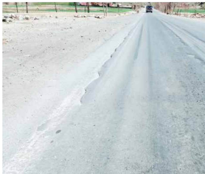
Rutting of the Pavement Surface
