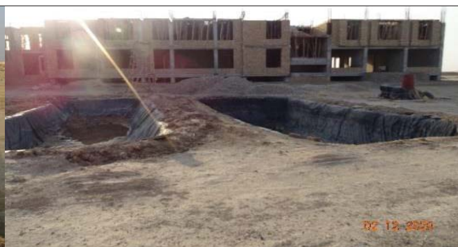
Poor safety and storage of materials at project site
