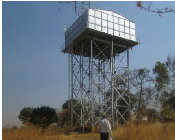
High Level Distribution Tank
