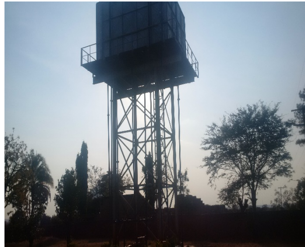
T2 High Level Supply Tank
