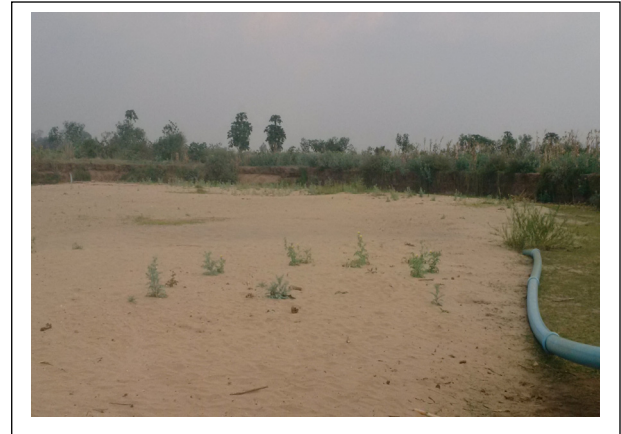
Main pipe washed away at Chapananga
