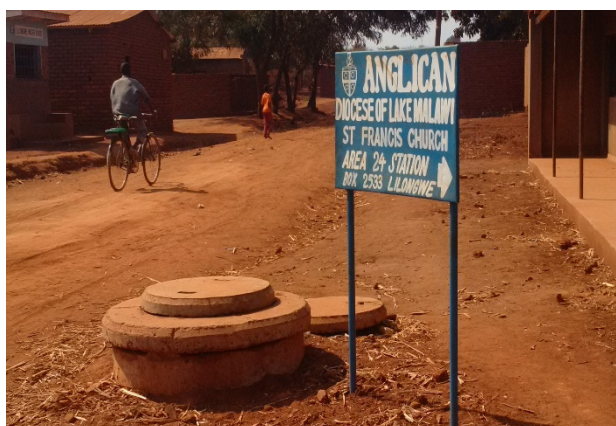
Valve Chamber at Area 24
