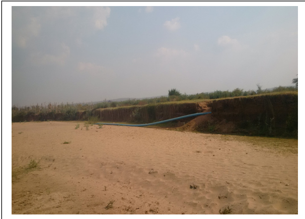
Main Pipe washed away at Chapananga
