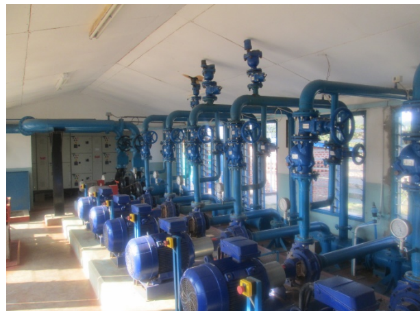
Pumps at Water Treatment Plant
