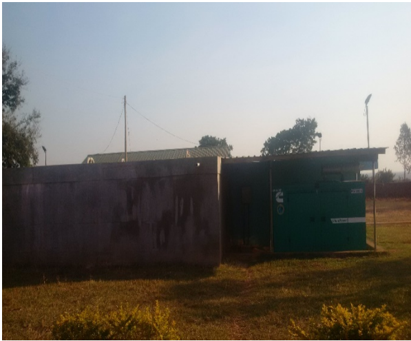
T2 Pumping Station Stand-by Generator & Tank
