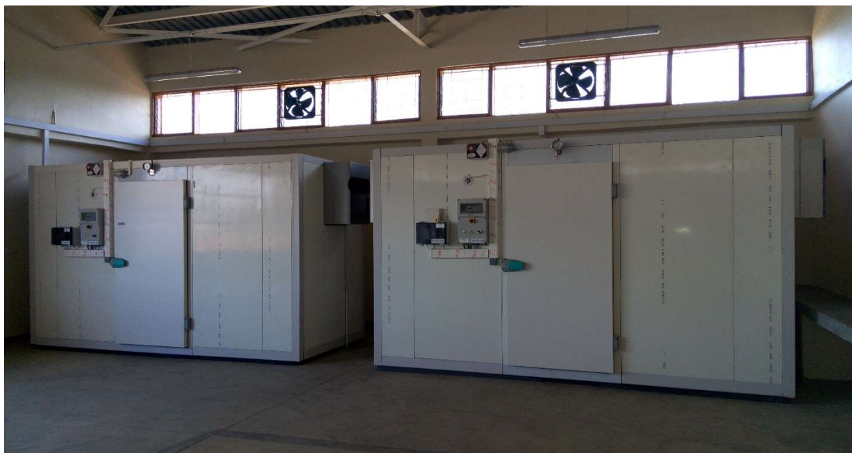
Picture 4.2.3.1 – Refrigeration Units in Cold Room
