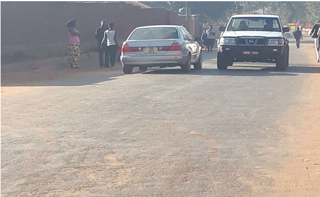
Photo 4.11.2 – Shows uneven road surfacing
