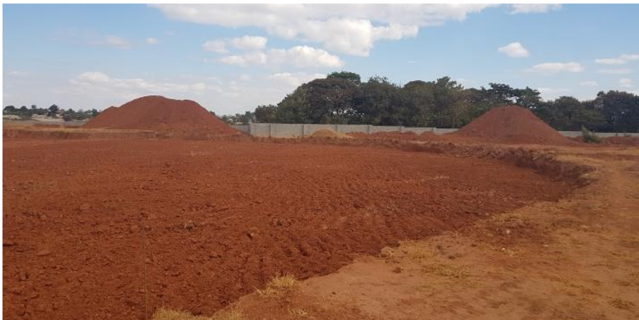
PICTURE 5.1.13—STALLED WORKS AT M'MBELWA STADIUM
