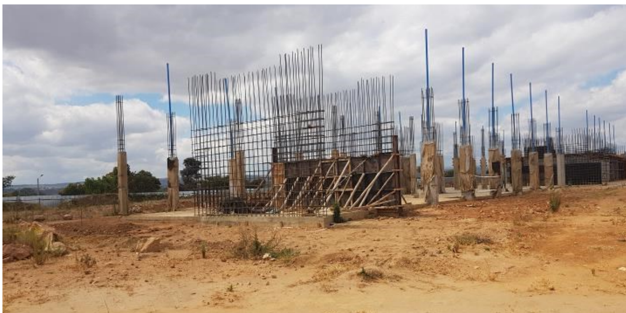
PICTURE 5.1.14—ABANDONED WORKS AT M'MBELWA OFFICE COMPLEX
