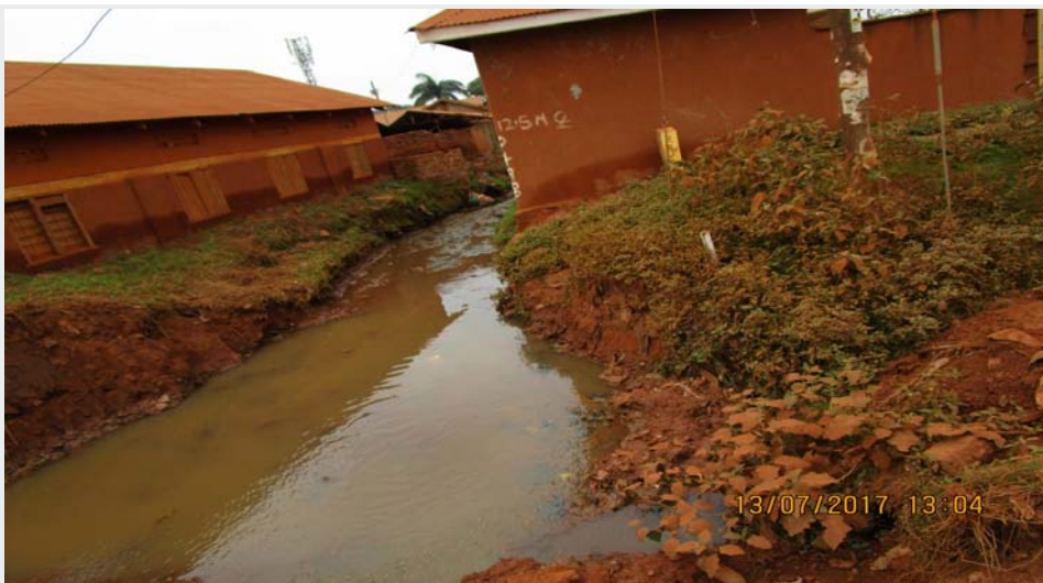
Figure 54: Outflow of water blocked by buildings.
