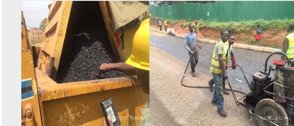
Figure 22: Safety issues at the site
