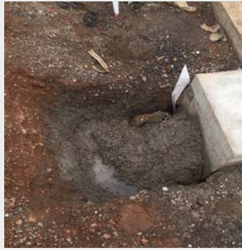
Figure 20: Uncompact concrete as backfill
