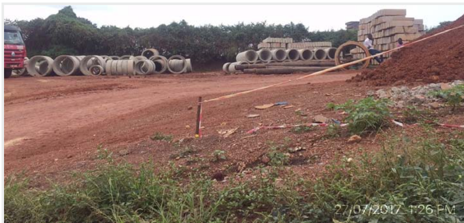
Figure 15: Stoke pile area unsecured
