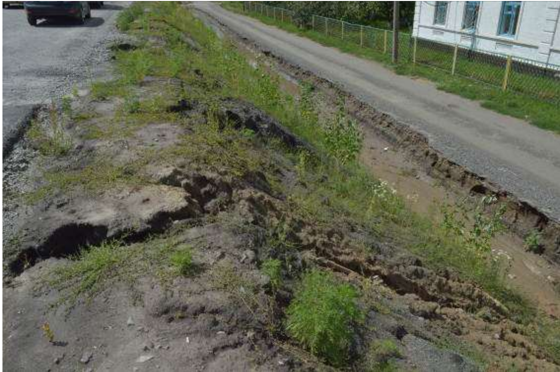
Figure 3 – Washaways in Podil village, km 288+794
