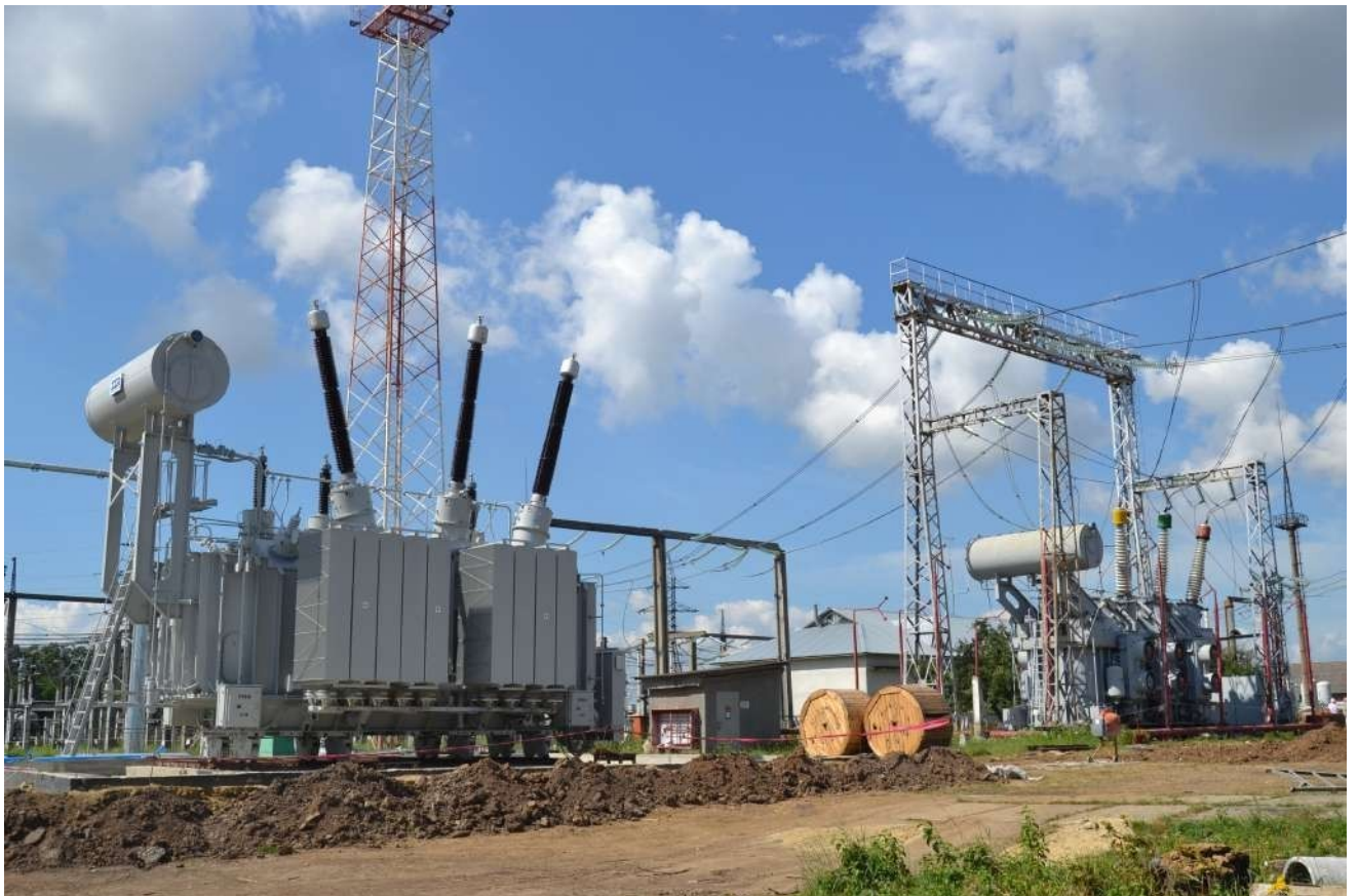
Photo 5: AT3 autotransformer installed at the design site (not yet busbar connected)
