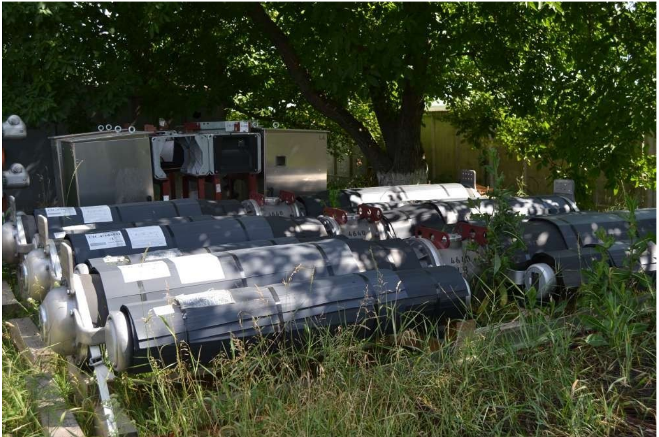
Photo 4: 330 kV gas-insulated switchgear manufactured by Siemens
