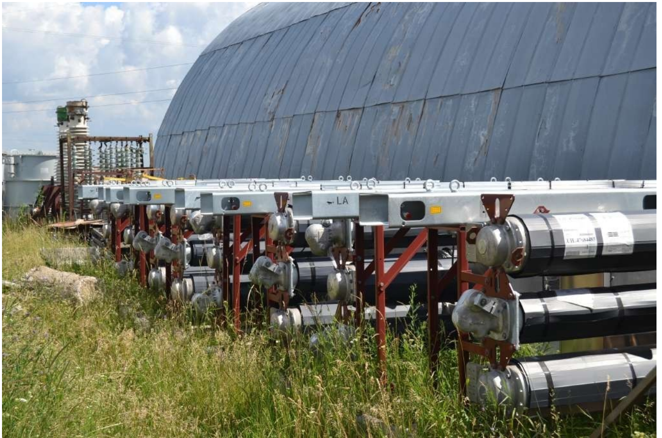
Photo 4: 110 kV gas-insulated switchgear manufactured by Siemens
