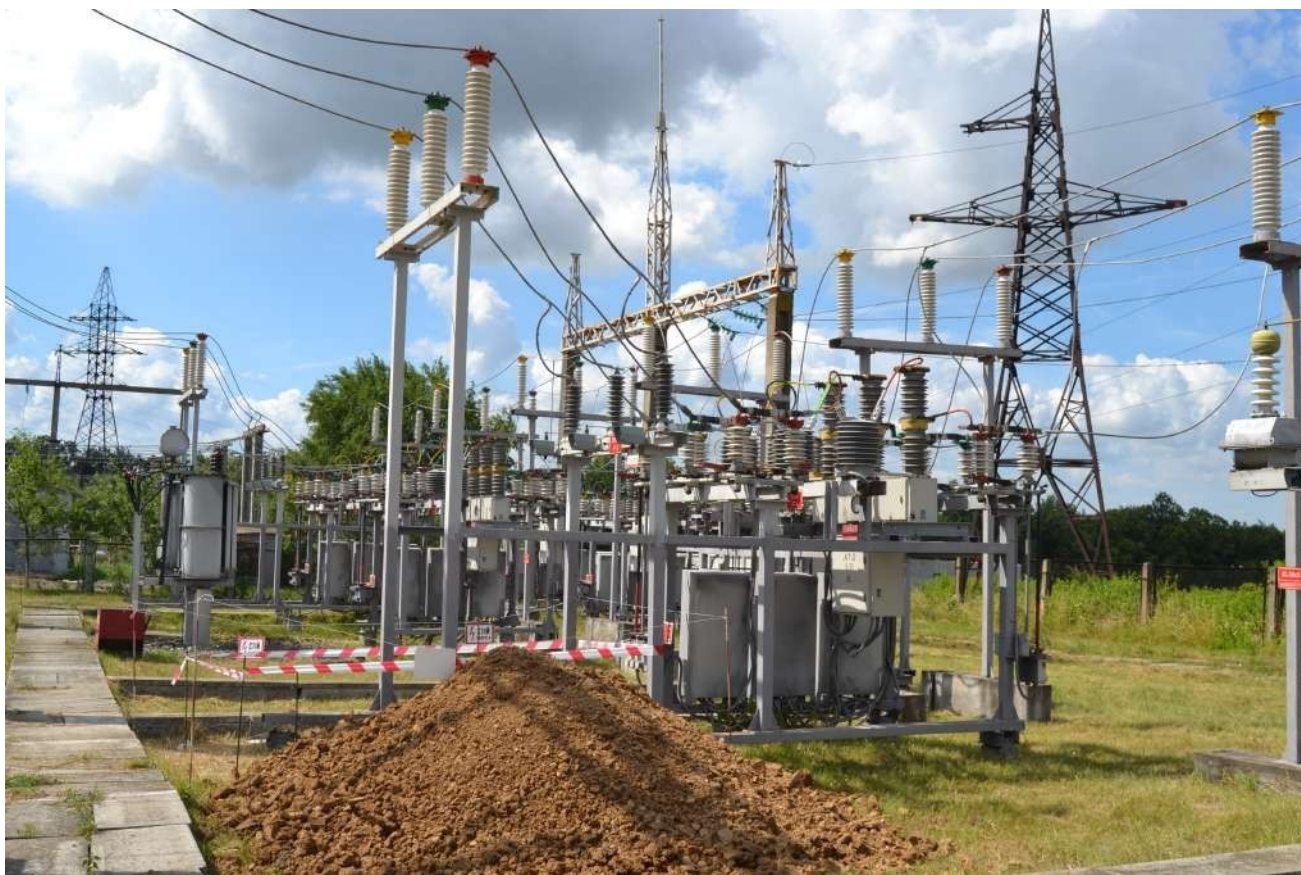
Photo 8: Fragment of the existing 35 kV VPR
